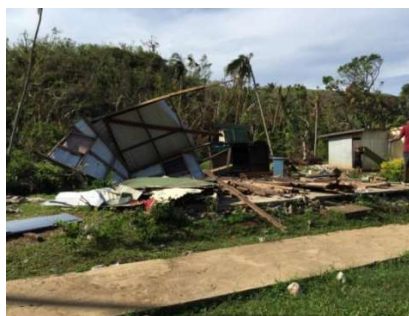
Nakorotubu District School Staff Quarters completely destroyed. Source: HLK Jacob. Cyclone Winston Preliminary Assessment.
